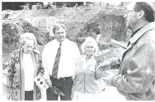
The laying of the first brick. From left: Mrs Meininger, Mr Scholefield, Mrs Strever and Mr Blight.
